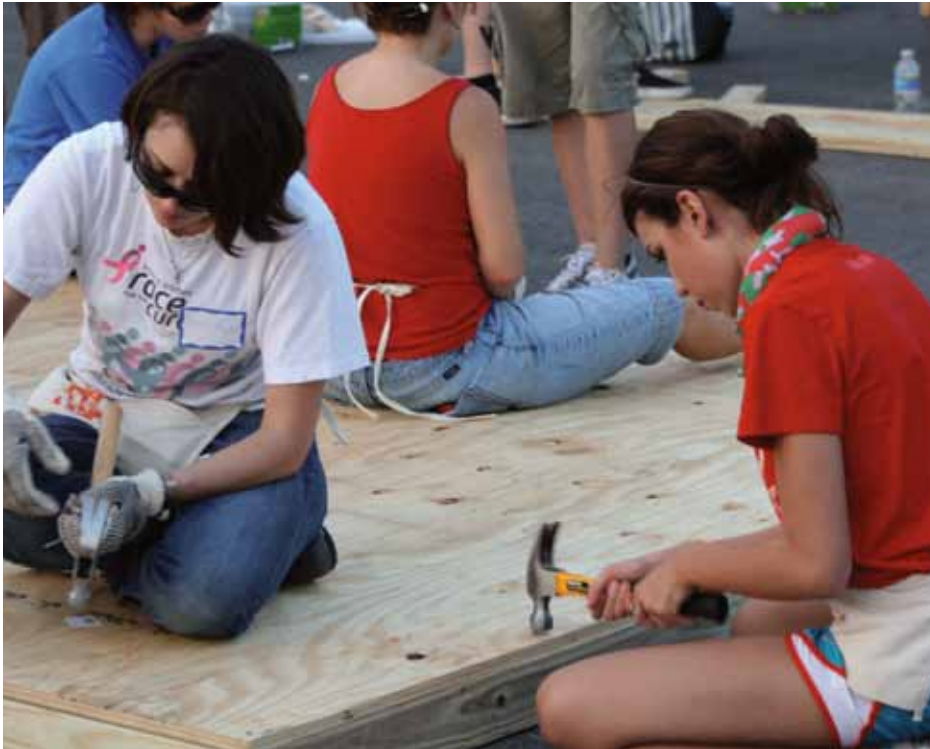
More than 800 volunteers from The U built 70 hurricane shelters in 50 hours. The shelters were shipped to Haiti to provide families with protection during hurricane season.
